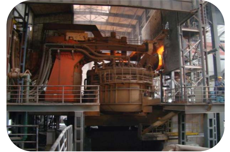
◆ 20t Electric-arc Furnace
